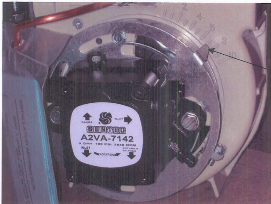
Air Shutter indicator (Beckett burner)
