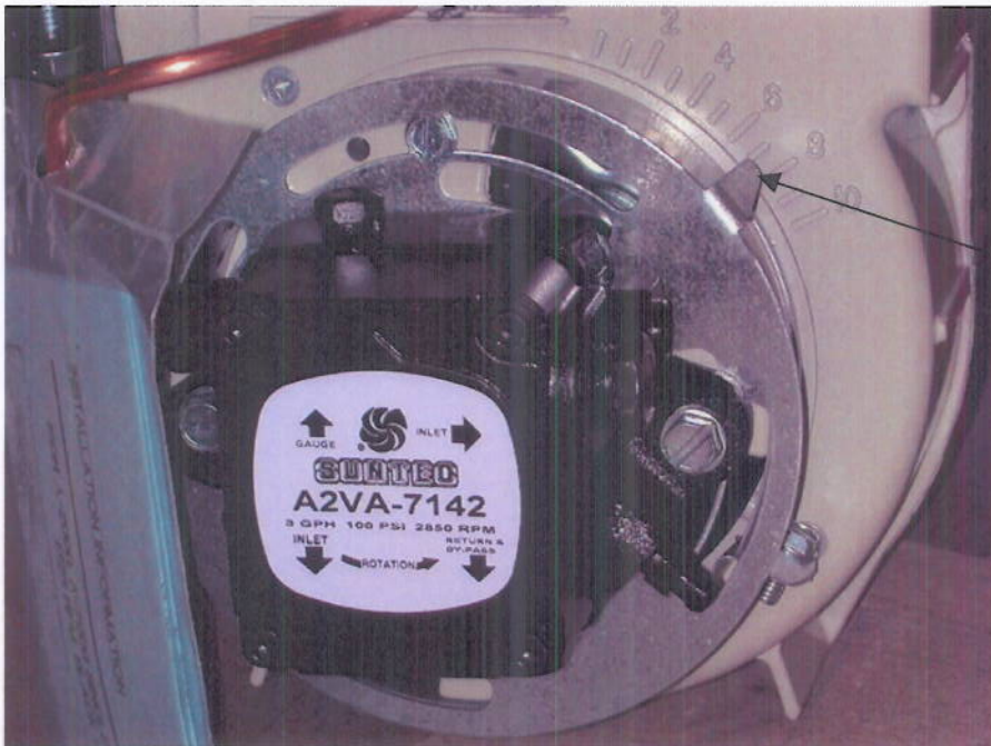
Air Shutter indicator (Beckett burner)
